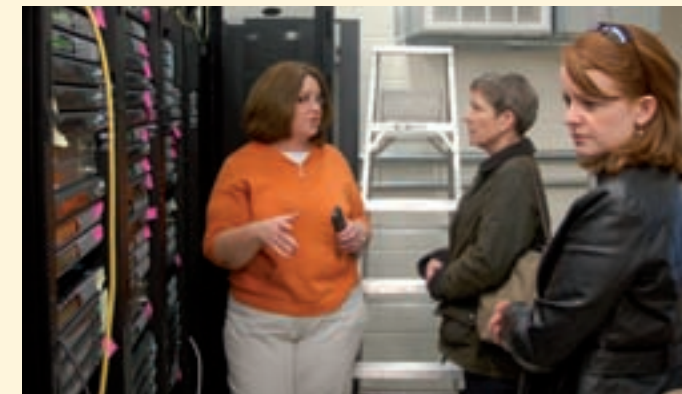
(Left to right) Hardy Fiber-to-the-Home Project Coordinator Becky Kimble demonstrates the company's OneNet TV equipment to new National Telecommunications Cooperative Association employees Barbara Fitzpatrick and Laura Withers.
