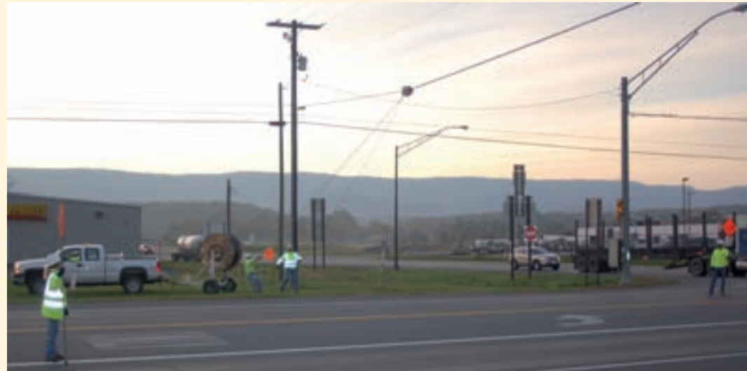
Above and below middle: Employees of ER Excavating & Utilities begin work on Hardy OneNet by placing fiber along U.S. 220 North in Moorefield.
