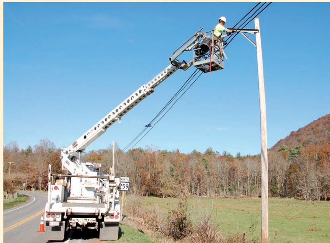
An employee of ER Excavating & Utilities, one of the contractors named to construct Hardy's AnchorRing network, places fiber November 2 along the intersection of W.Va. 259 and Kimseys Run Road.
